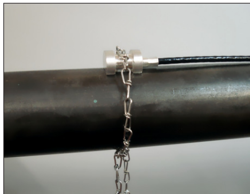
PT100 sensor fixed to pipe
