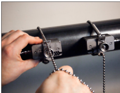
Transducers mounted using clips and chains
